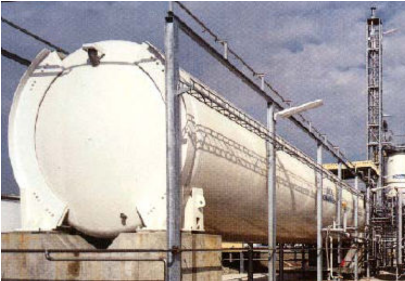
Figure B-22: Liquid hydrogen storage of Linde AG in Ingolstadt, Germany (Source: Schmidtchen (2003)).
